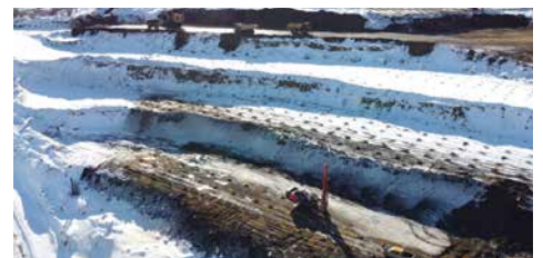
Business partner Kiewit is on-site and continues completing the main mine road, water-catchment systems, and the infrastructure and ore load-out pads. Most of Kiewit's construction work is complete.
