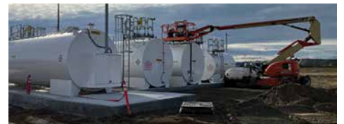
General contractor Conam is nearing completion of construction work. This includes completion of the communication tower, liner work and the fuel island.
