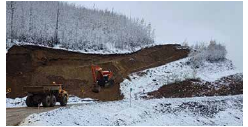
Project business partner Qayaq finished the mine access road. Qayaq is now working on several punch-list items, such as slope stability and berms along the road.
